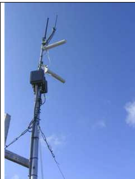
Repeaters on San Patricio Hill
