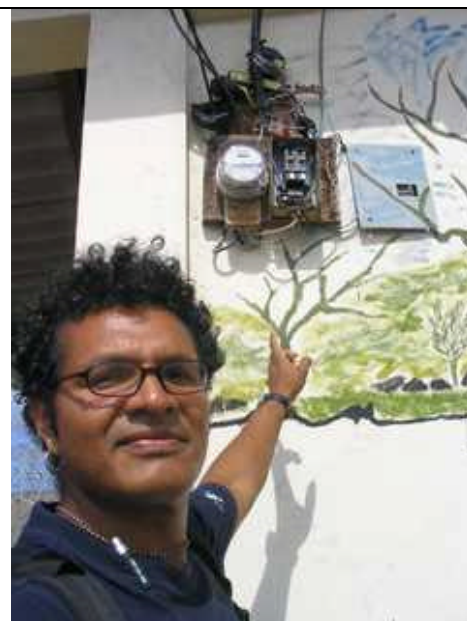
Energy monitoring at Colegio
